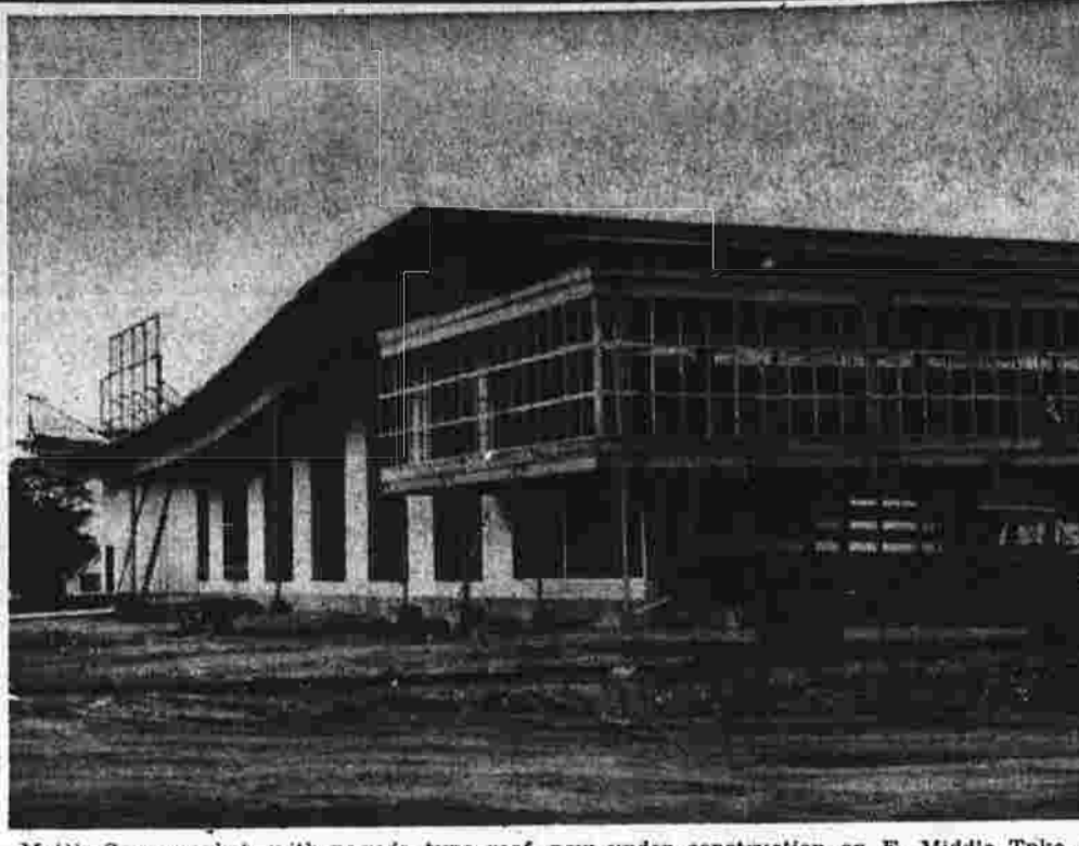
Mott's Supermarket, with pagoda type roof, now under construction on E. Middle Tpke. near Vernon St. will present a unique public auditorium in mezzanine addition (foreground). The new 21,000 square foot, two level floor area plus mezzanine (first of its kind in Manchester), is expected to be completed in late September or early October. (Herald photo by Saterini).
